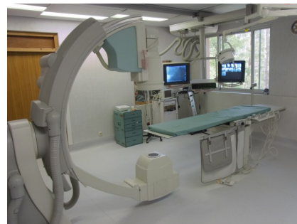
A new Cath lab is installed in a hospital in Nepal thanks to RAWCS
